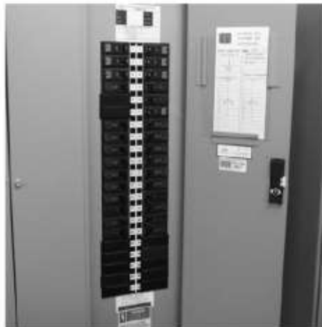
Figura 2.10: Panel de Breakers
